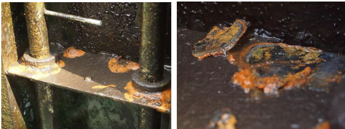
Edelstahlblech in WWZ
